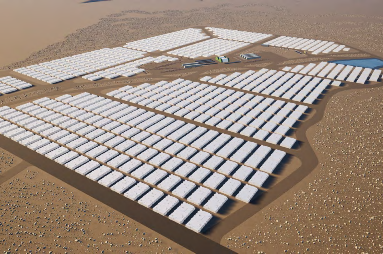
Overhead View of Battery Storage Facility
