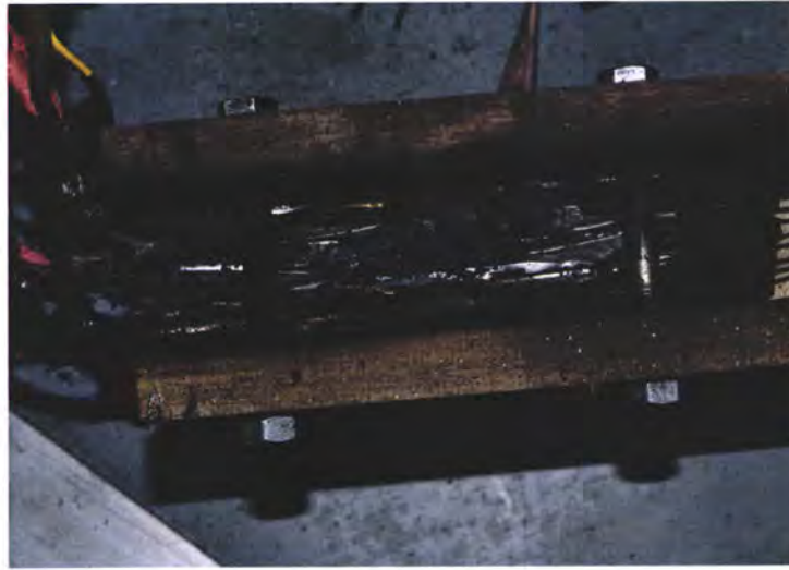
Figure 11. Photograph of the 5S1P battery post-propagation test initiated at the center cell (Cell 3).
